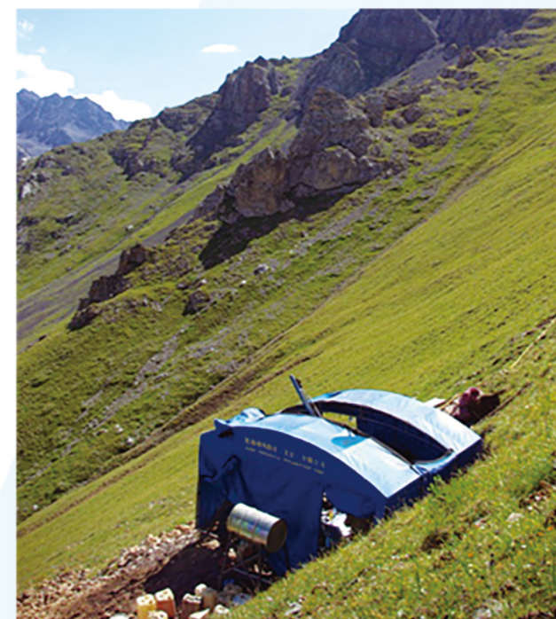
XDY600P便携式岩心钻机在内蒙古施工 XDY600P Working site in Neimenggu
